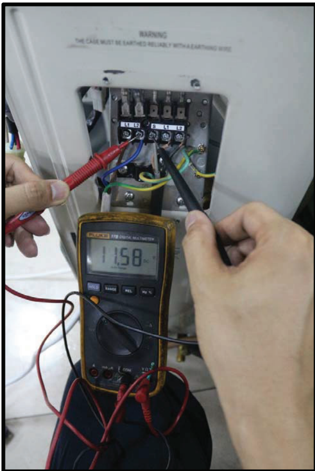
Fig. 30 – Test the DC voltage
