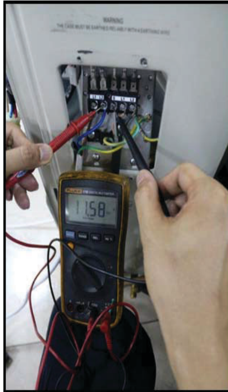
Fig. 23 —Test the DC voltage
