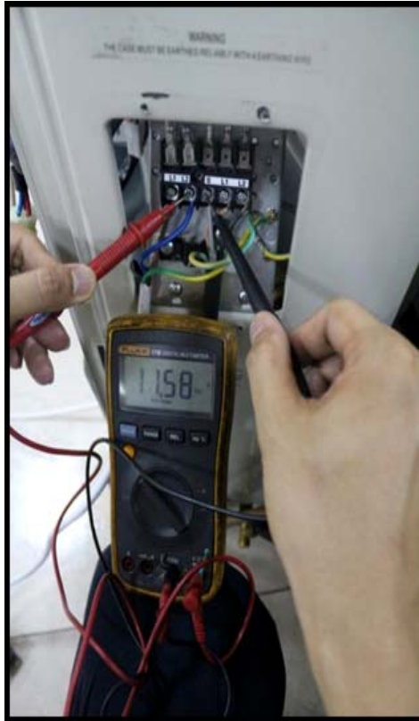
Fig. 23 – Test the DC Voltage
